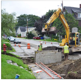
photo by Vanessa Fournier An excavator from Munson Earth Moving Corp. of Williston lowers a trench box for working on installing a new jet hydrant Friday. This was the last of the main waterline installations for Church Street, Maple Street, Slapp Hill and Vermont Avenue. Spot paving is scheduled to begin this week.
