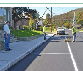
Hardwick Town Manager Jon Jewett (left) watches as Tom Badkins (right) and Percy Allen (center) of the Public Works Dept. crew paint parallel parking spaces in front of the Hardwick Elementary School. The select board voted to change the parking from angle parking for safety reasons.
