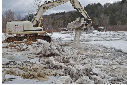
photo by Vanessa Fournier Gary Bellevance of Bellevance Constructors, Inc. opens up a channel at the end of Christies Street in Hardwick, Vermont. The curved pipe cut at the water back to the Cottage Street Bridge so the water could flow more freely.
