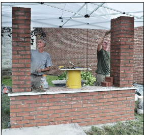
Jim Nevins (left) and Karl Armstrong (right) of Armstrong Meadows of Lyndonville built a 7-foot high by 9-foot wide brick sign Aug. 6 in front of the Vermont Elementary School. The sign, which is electrically operated, says again will be controlled from inside the school.
