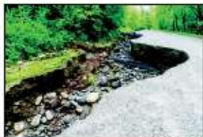
What is left of the old Northwestern Road in Greenboro, Vermont. The road was destroyed by a portion of the wall.
