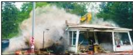
On August 12, 11:30 AM the top floor of what remained of the Carr House collapsed into the street. The house could not be salvaged in a way that would allow it to be used as a museum. Photo by Doug McClure.
