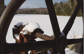
This gate operating system mounted on the aqueduct supplying the East Long Pond. The dam is owned by the New York State Department and is considered to be a poor option by the State of Vermont.
